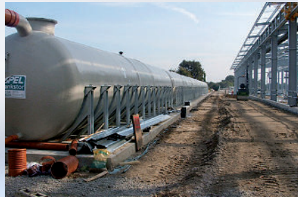
SPEL Tankstor® rainwater attenuation scheme at the Ramsgate Traincare facility. Five, 400 Series 85,000 litre capacity.
