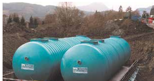
SPEL Septic Tanks 600 Series 200,000 litre Kinlochard WWTW, Aberfoyle
