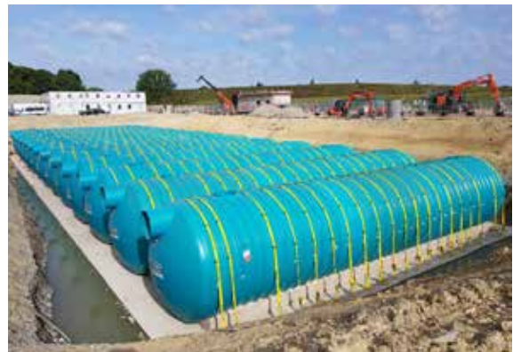
Boing at Gatwick Airport, thirteen 600 series 4m dia. tanks totalling 3.1 million litres capacity
