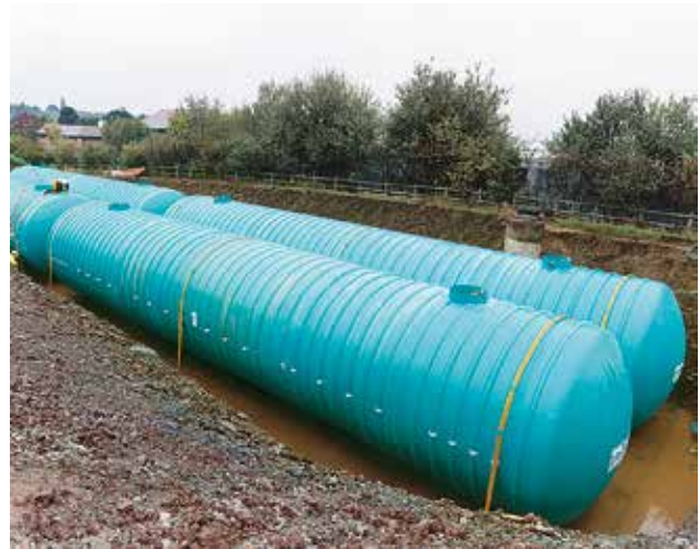
Eight SPEL Tankstor® 600 series Stormwater attenuation tanks have been installed at Buntsford Hill, Bromsgrove to provide 2,100m 3 of capacity
